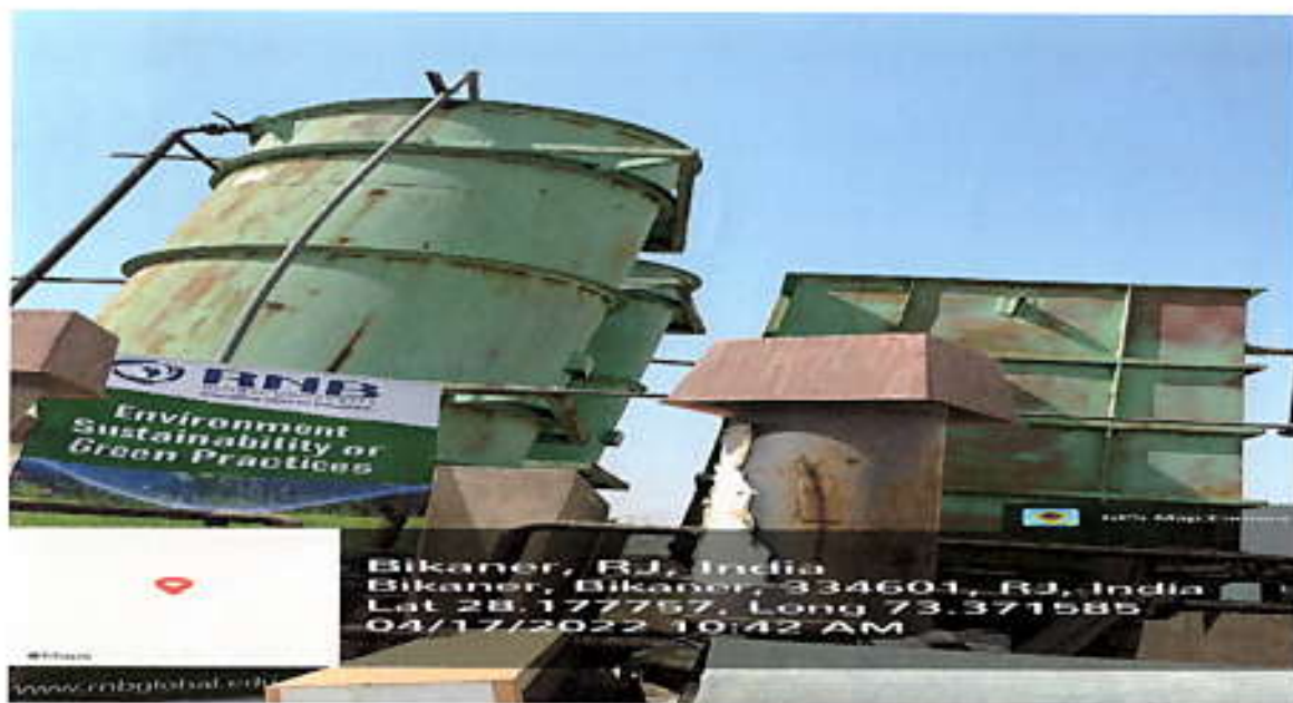
Sewerage Treatment Plant at RNBGU
